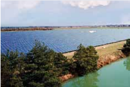
7.4 MW solar power plant, Nordendorf, Germany
