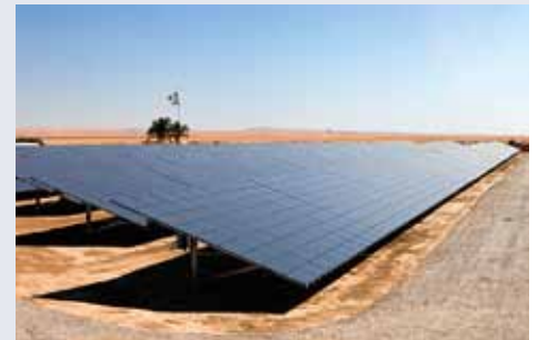
1.2 MW installation in Coalinga, California
