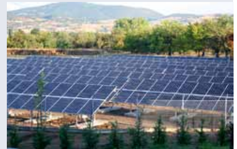
Also reliable in salty sea air: solar power plant in Greece, 100 kWp
