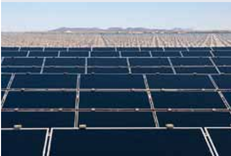
290 MW (AC) Agua Caliente solar PV plant under construction in Yuma County, Arizona, USA
