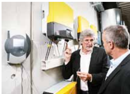
String inverters with monitoring system
