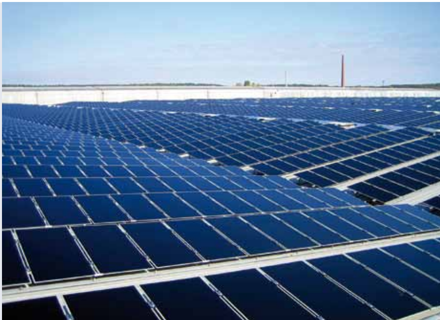
64,000 thin-film modules on 193,000 m 2 : roof-top installation in Hassleben (Germany) with a capacity of 4.64 MW
