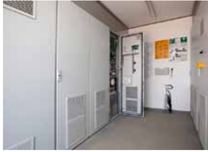
Left: Central inverter
