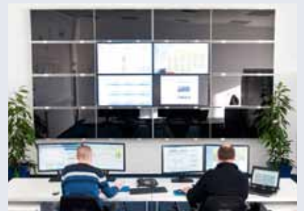
Control center with real-time power plant management system
