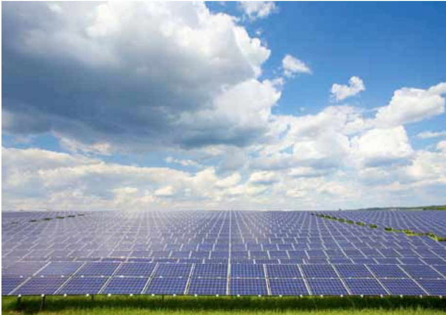
A 14.37 MW solar park with 62,766 modules installed on around 28 acres in Richelbach
