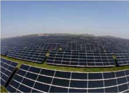
Left and below: Solarpark Waldpolenz (Germany)
