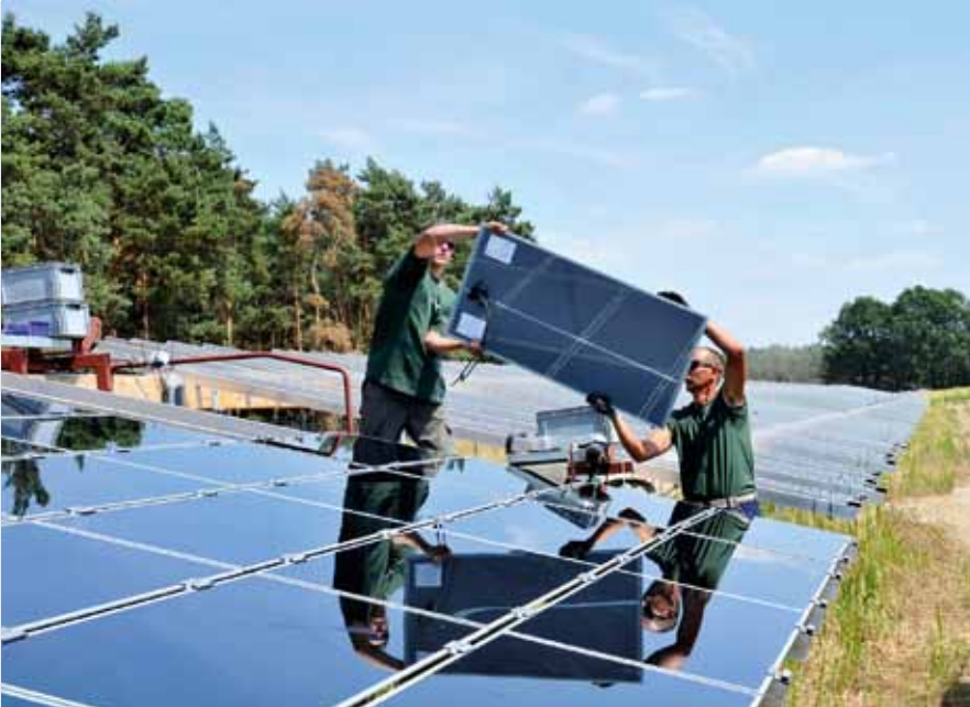
BELECTRIC's own construction team members installing solar modules in California, USA (below)
