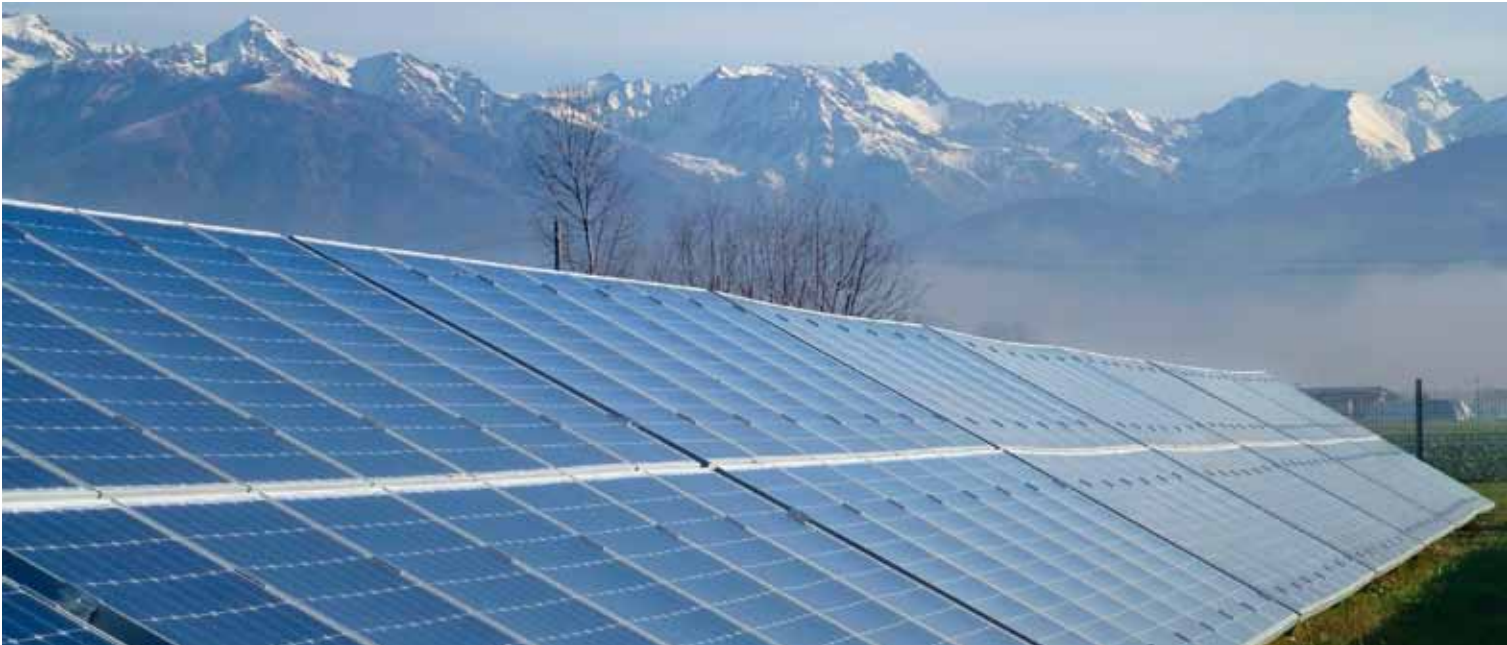
1 MW solar park in Villafranca (Italy) with PerfectEnergy modules
