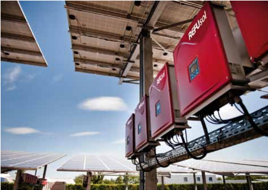
REFUsol string inverters at 4.6 MW PV installation in Belgium
