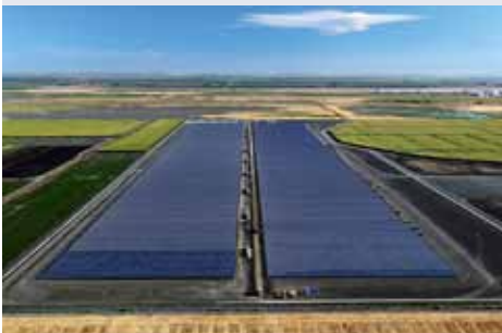
20 MW solar field with AE inverters
