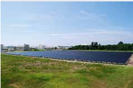
1 MW system in Niigata, Japan's 1st commercial solar power plant
