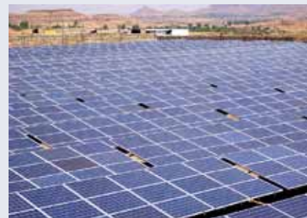
In Itnal (India) 13,000 solar modules produce over 4,000 megawatt hours of clean energy each year.
