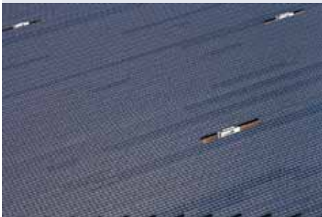
The photovoltaic plant in Ravenna, Italy, 124 MW with Santerno Sunway Stations
