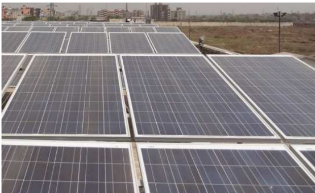
Large Solar Photovoltaic project
