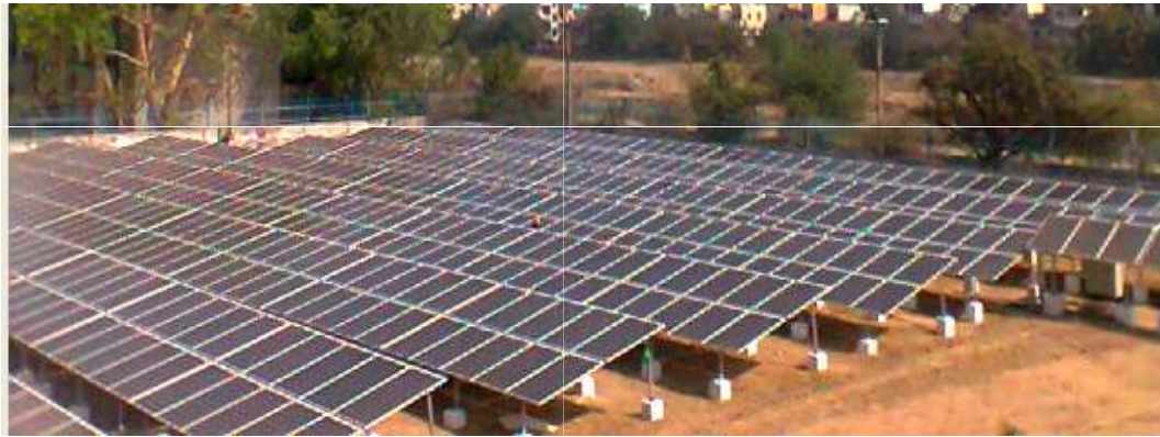
225 kWp Solar Photovoltaic project
