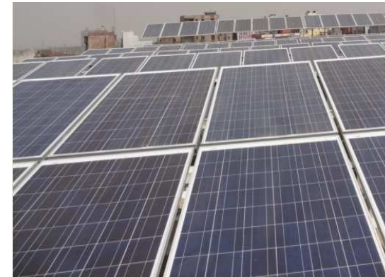
55 kWp Solar Photovoltaic project
