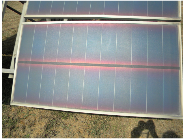
Figure 4.1 CIS modules under field condition
